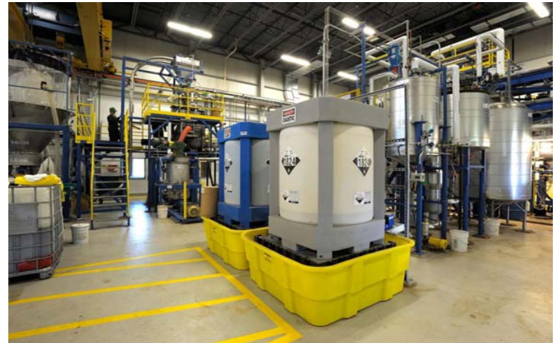
Biofine Gorham, ME pilot plant
